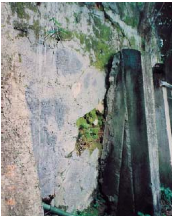
(c) Cracked Surfacing on Rubble Wall
