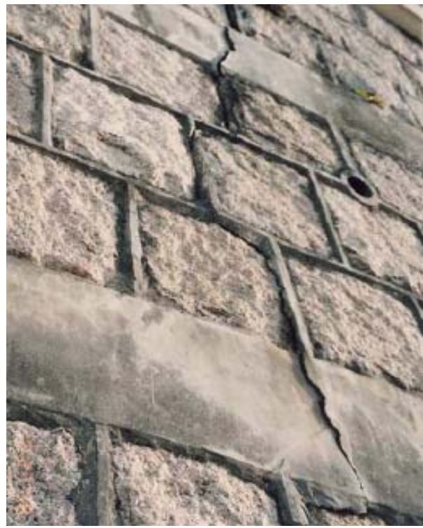
(b) Crack in Retaining Structure
